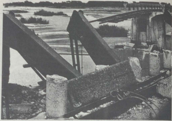
A Mozambican bridge destroyed in a South African attack
